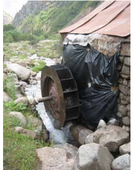
Most of the improvised micro hydro plants are made out of spare parts and are quite inefficient.
